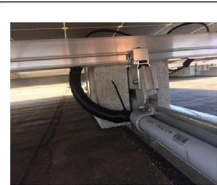
PHOTO #5: Row to row DC wiring can be pulled through PVC conduit attached to the base rail and split loom wire protection.
