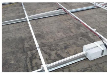
PHOTO #1: East West rails can be used to secure PV wire. In this image, the installer has used PVC straps secure on the rail to support the PV wire.
